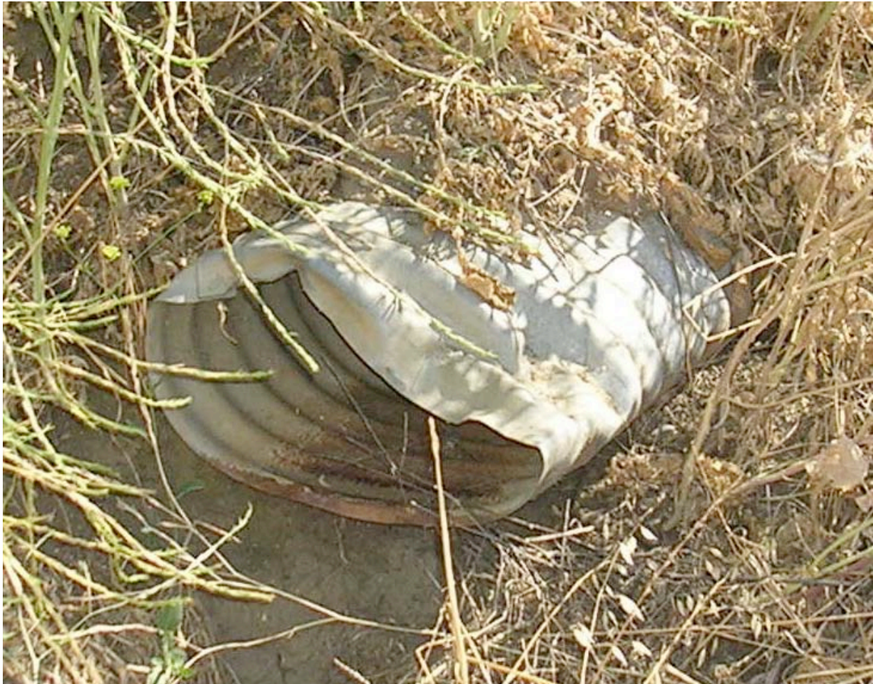
Undersized aging culvert onto Vigna Farm June 2005
